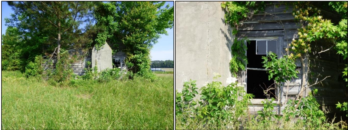
Photo 38: Tenant House Rear Ell Addition, Southeast Elevation (Left) and Detail of Wood-Frame Window on Rear-Ell Addition (Right).
