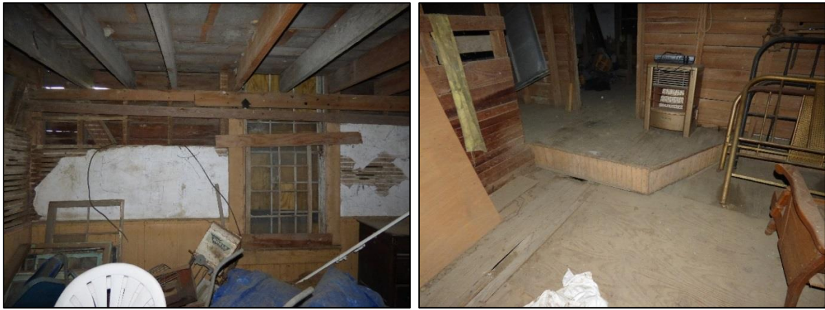
Photo 94: Exposed Lathing and Boarded Window (Left); Pulpit Addition (Right).
