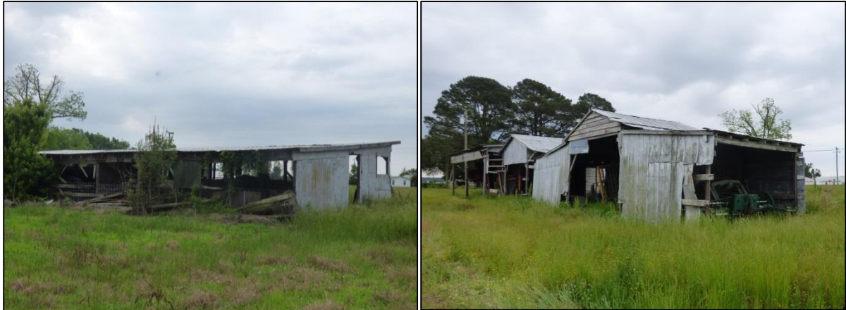
Photo 88: Machine Shed (Left) and Cluster of Outbuildings (Right) within Church Cross Roads.
