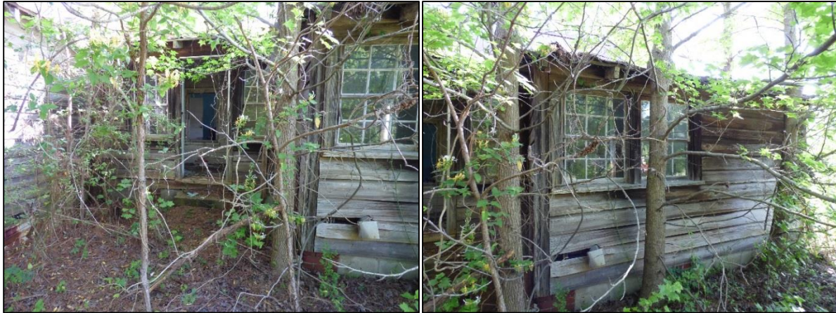
Photo 39: Multiple Shed-Roof Additions Extend Off of the Rear-Elk Addition of the H. A. Bowen Tenant House.
