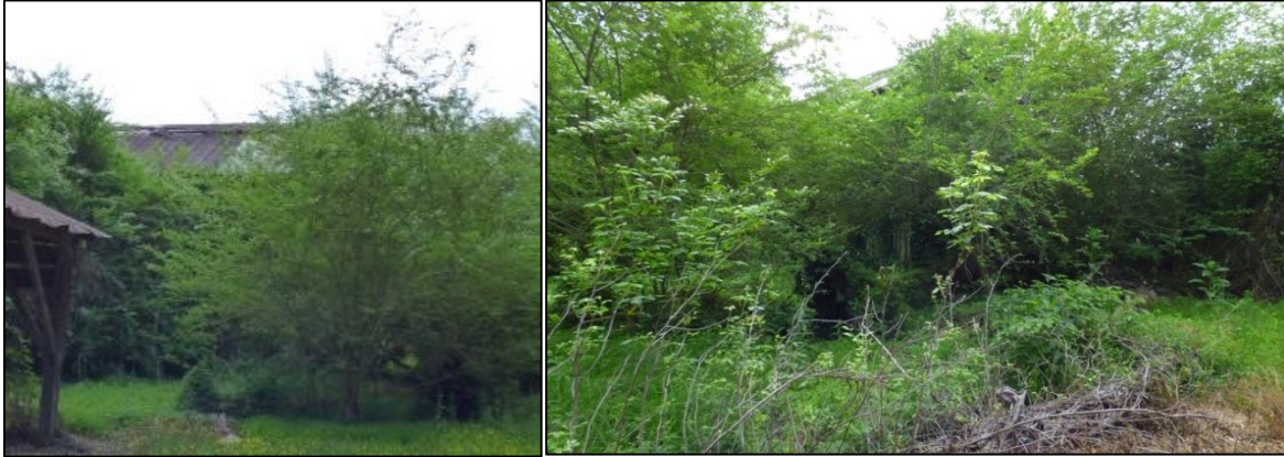
Photo 131: Outbuilding Overgrown with Vegetation, North Elevation (Left) and Northwest Oblique (Right).
