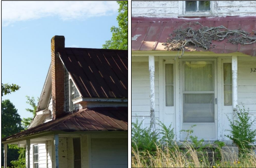
Photo 12: Detail of Chimney on Northeast Elevation (Left) and Detail of Primary Entrance on Northwest Elevation (Right).
