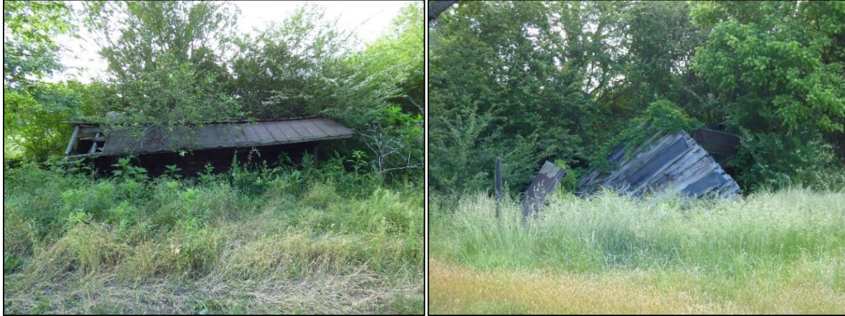
Photo 16: Collapsed Machine Shed (Left) and a Collapsed Possible Tobacco Barn (Right).
