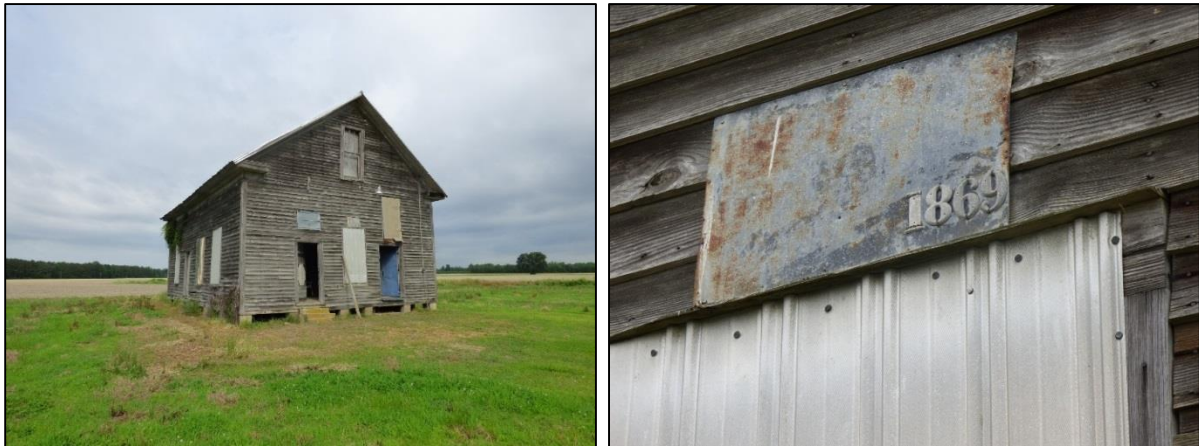
Photo 91: Primary Resource, Southeast Oblique (Left); Detail on Façade of Primary Resource (Right).
